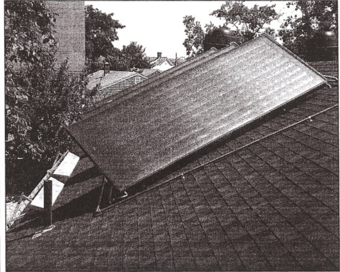
SOLAR PANELS WILL PROVIDE HOT WATER FOR RESTAURANT.
