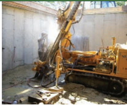
LEFT: The geology of the site made for a challenging geothermal installation.
